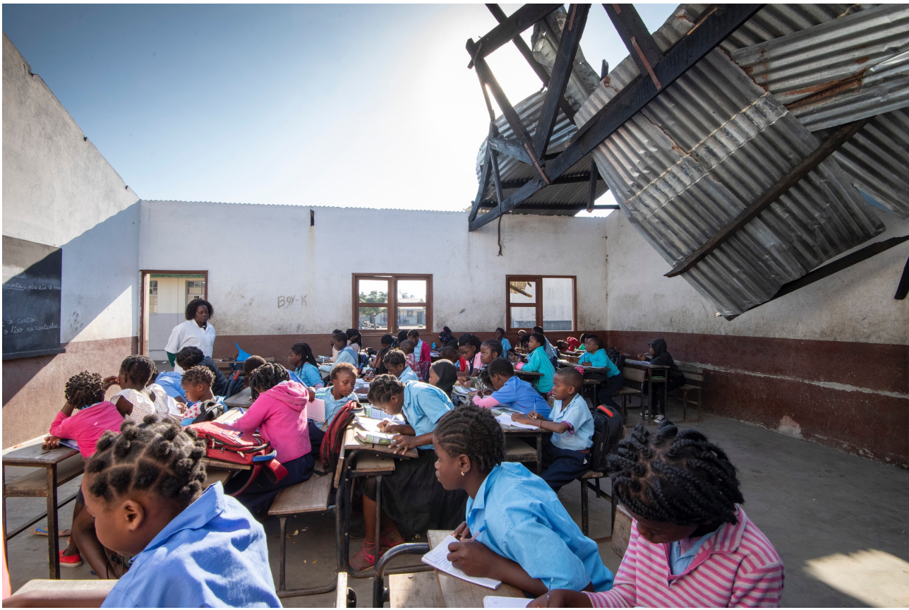
Figure 2: Images of infrastructure damage and impacts of tropical storm events
